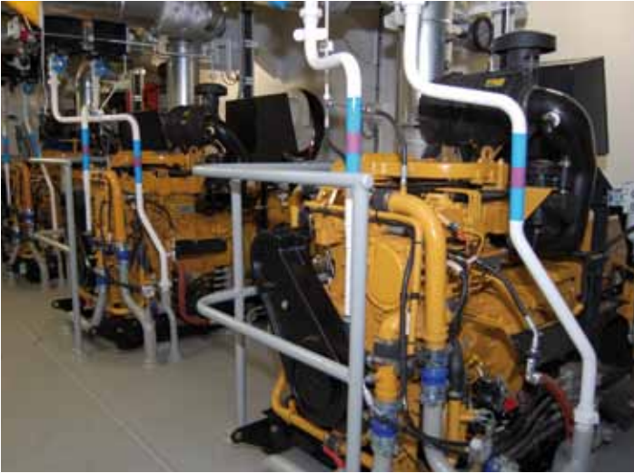
During normal service, one of the three generators is running
